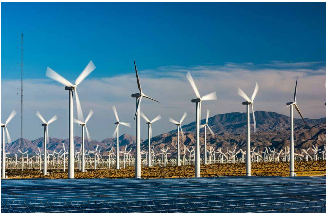
Wind Turbine Farm and Solar Panels, Southern California
